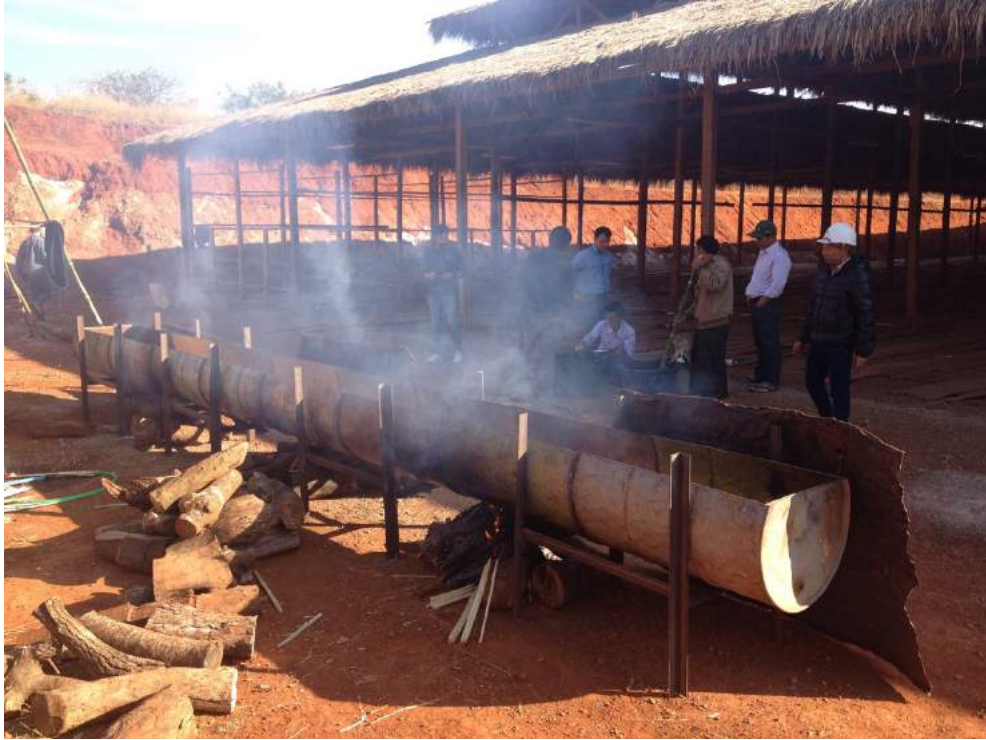
Borax Treatment Tank with fire for Hot Method
